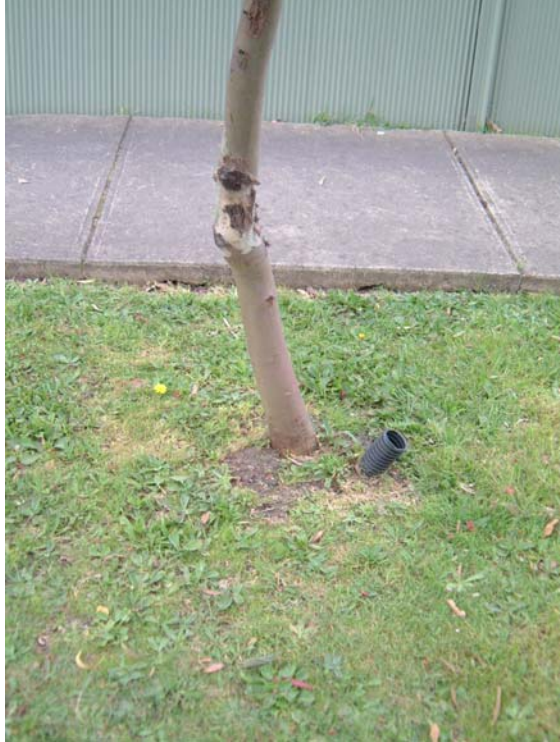
Close view shows the nature strip well below the pavement surface.
